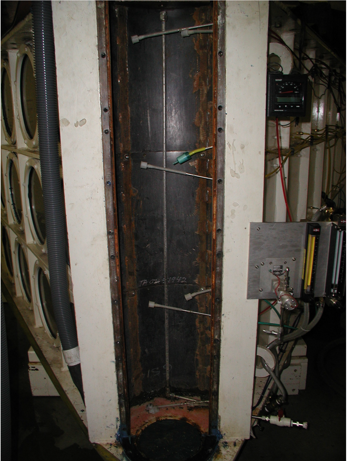
Photo A4.7 – Screen Removed
