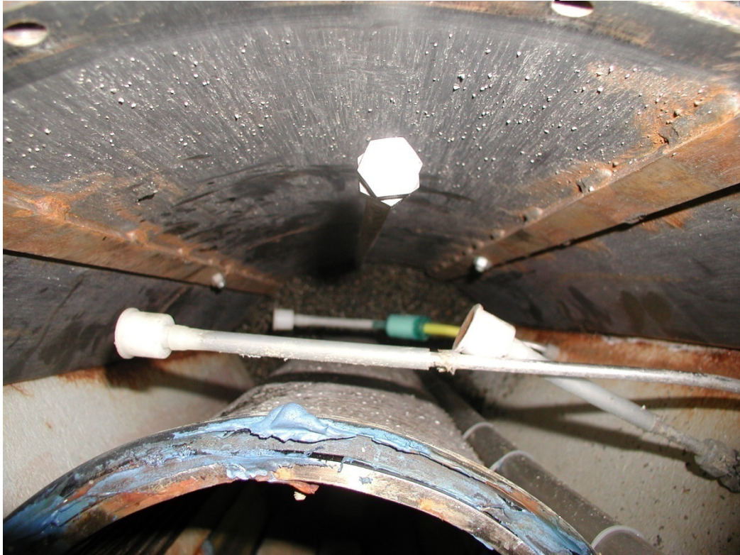
Photo A4.6 – Filter Pack Divider Close Up
